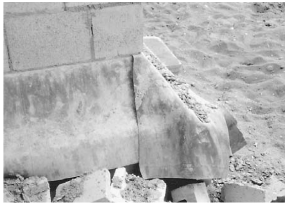
Figure 15-26 Unsealed lap joints allow water to circumvent the flashing.
